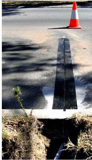
BL Sensor installed, ready to be encapsulated
